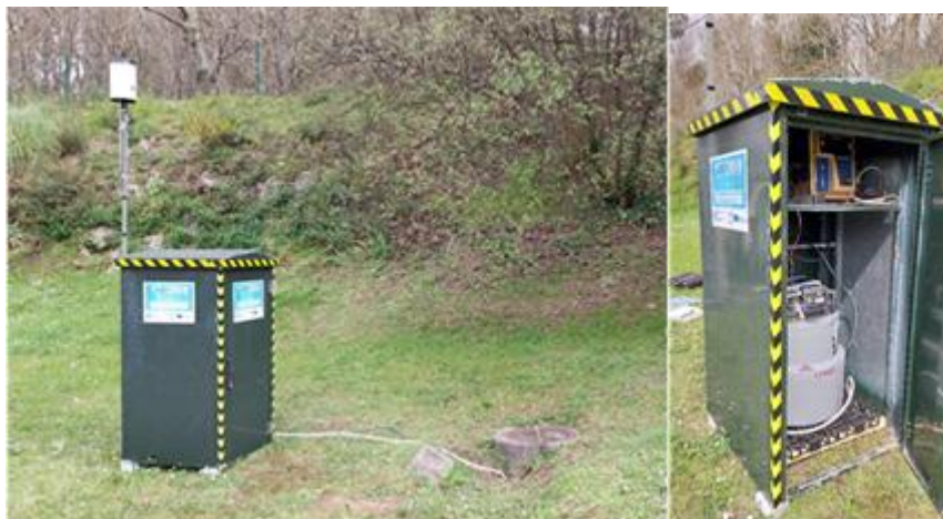
Figure 28: Stormwater sampling station with monitoring equipment, flowmeter, data loggers and power supply batteries
