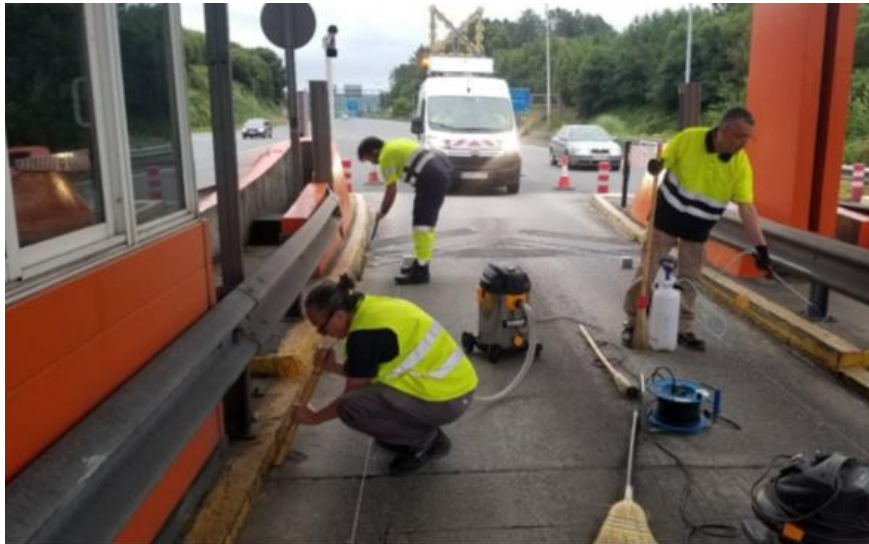
Figure 25: Development of sweeping/ vacuuming operations on lane 2 of the AP9 toll station at Cecebre.
